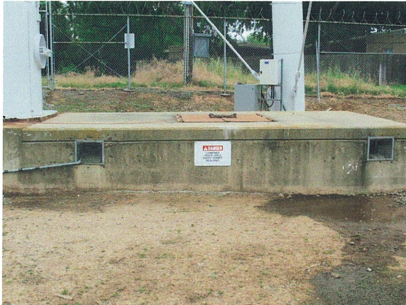
Underground valve vault where pressure gauges were formerly located.
