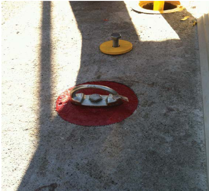
PowerSert, High Performance, drop-in anchor ($62) installed into concrete walkway using HIT-RE 500 SD epoxy ($50) created an anchor point for fall restraint system. Brackets are removed when not in use and are flush with surface.
