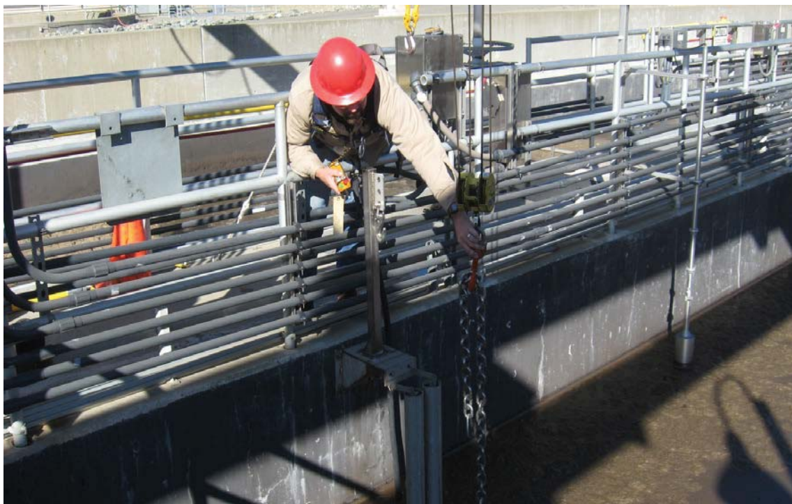
Staff safely connects hoist to pump lift chain to remove from aeration basis to perform maintenance.
